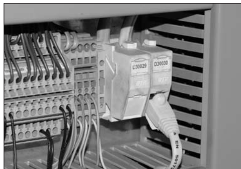
Application: E-DAT modul REG 8(8) IP20 installed in a machine distributor
